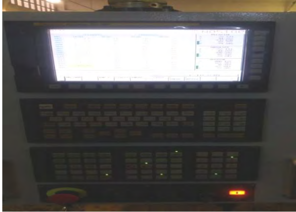
Figure 5. Fanuc equipment control panel
